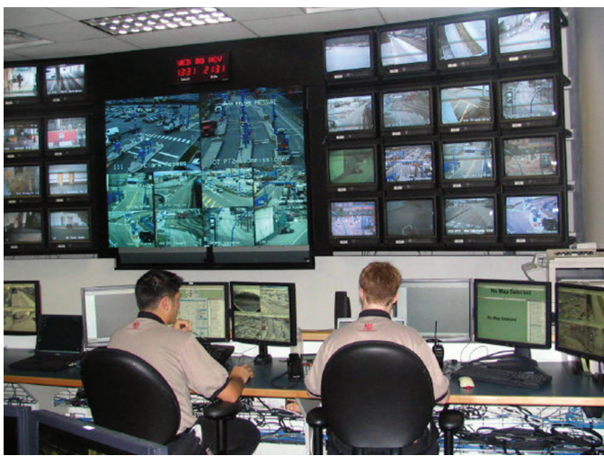
Eyes in the sky — the security control room at the Vancouver Port Authority. The perimeter of the Port is monitored through state-of-the-art digital telescopic cameras and software that can scan details of vehicles and individuals.
